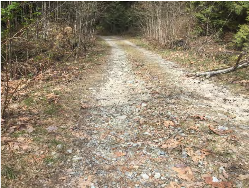
No downstream curb log and gap in surfacing
